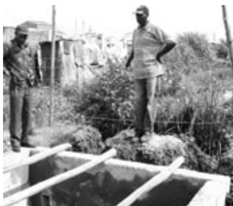
An underway toilet construction in one of the in-formal schools in Nairobi slums.
